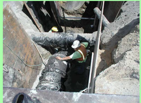
Vertical offset of a 24-inch ductile iron water main to accommodate an existing 12-inch main.
